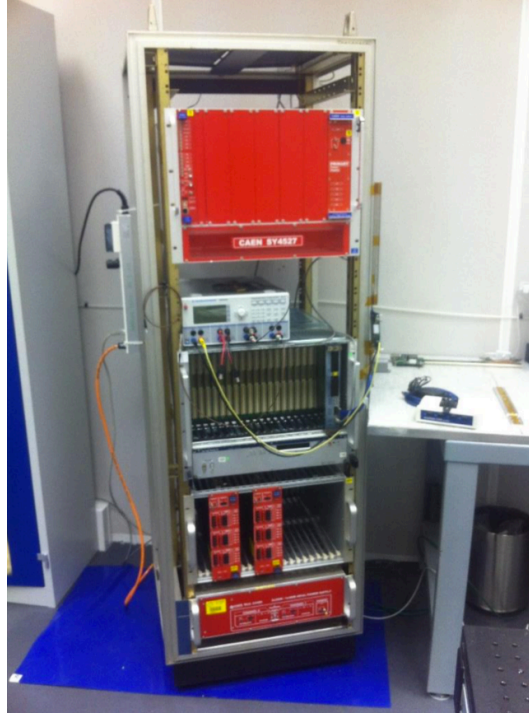
Figure 4.1: The test bench of the CAEN power supply system for the MFT constructed by K. Yamakawa [39]
